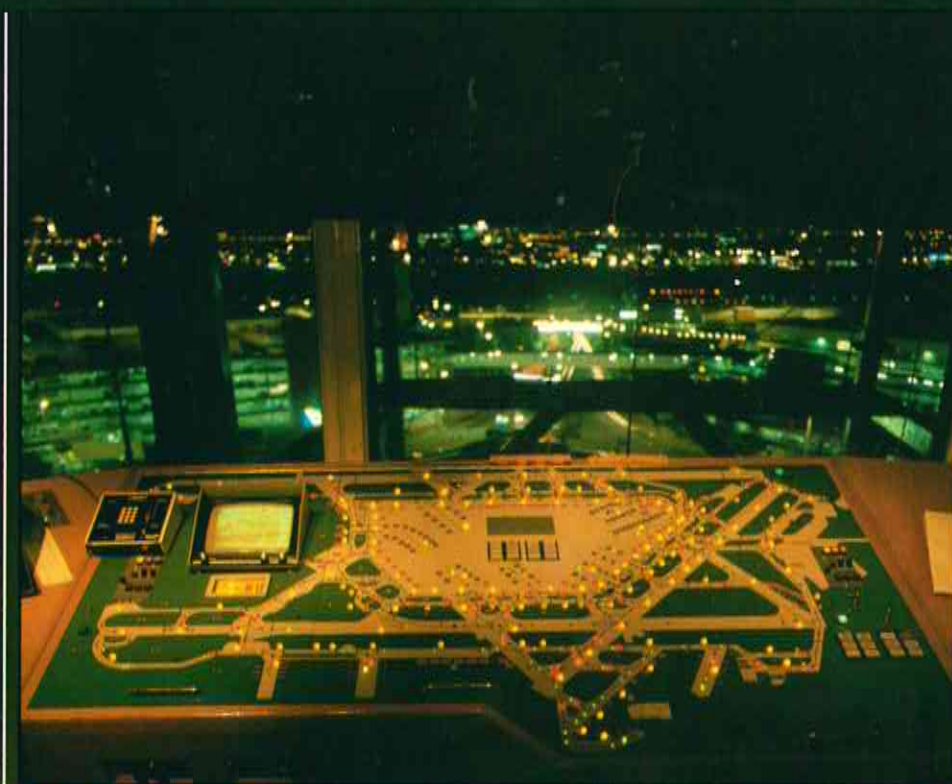
The Lighting Control Panel
