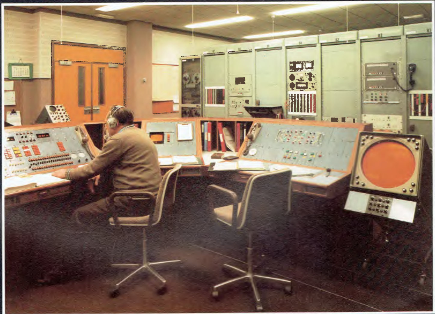
Telecommunications equipment room ▶
